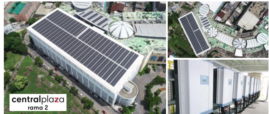
CPN at Central Plaza Rama II 998.8 kWp
