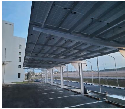
Southern Industrial Estate Songkhla Provincial (SEZ) 42 KwP
