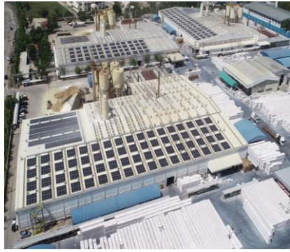
Quality Construction Products Public Co., Ltd. (Q-Con) 265.44 kWp
