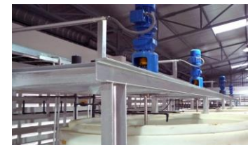
Water Treatment & Water reuse
