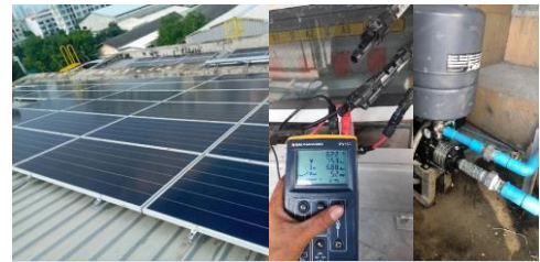
My Press Solar Roof 78.72 kWp
