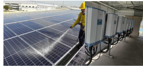
Siam Toppan Solar Roof 859 kWp
