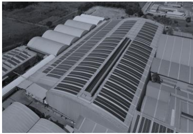
Solar Cell : 13 MW as of Dec 2022
