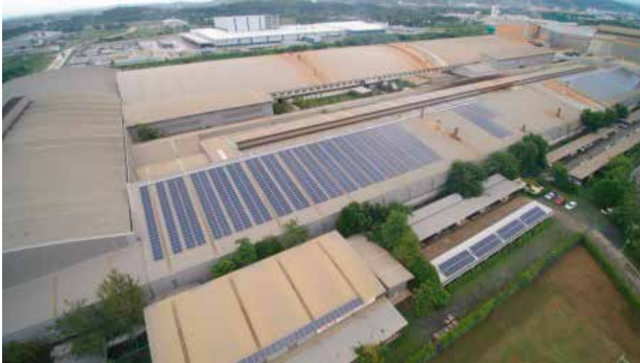
PV Solar Rooftop, 1.8 MW capacity, at Nong Khae Industrial Estate.
