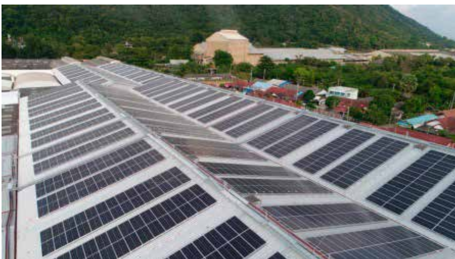
PV Solar Rooftop, 2.0 MW capacity, at Hin Gong Plant.
