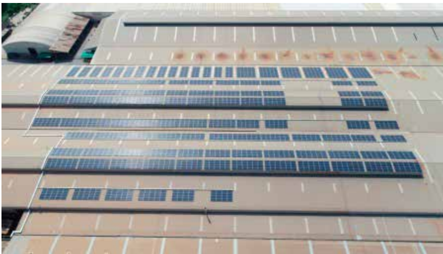
PV Solar Rooftop, 0.9 MW capacity, at Nong Khae Plant No. 1
