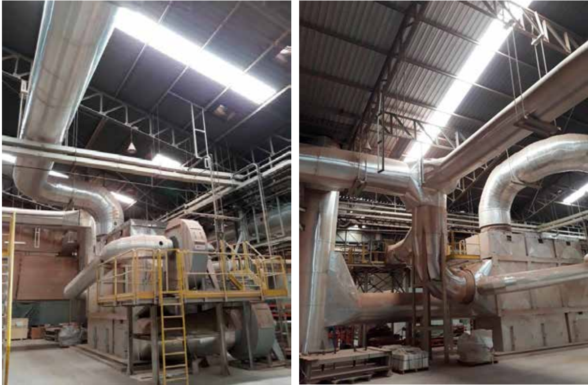
ระบบ Waste Heat Recovery from Kiln's Chimney (Air to Air Heat Exchanger)
