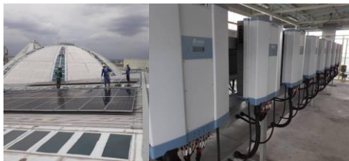
Central RAMA II Solar Roof 999.19 kWp
