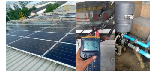
My Press Solar Roof 78.72 kWp
