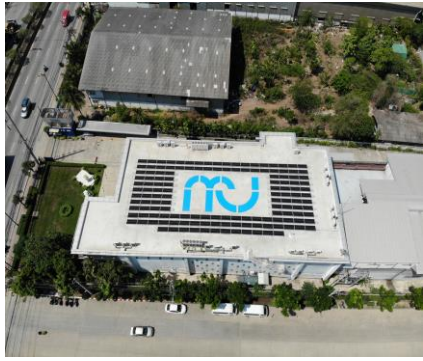
M.J. Bangkok Valve & Fitting Co., Ltd 56 KwP
