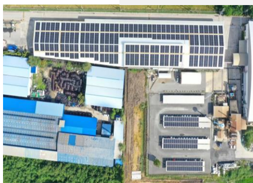
SCG Packaging Company Limited Solar Roof 999.6 kWp
