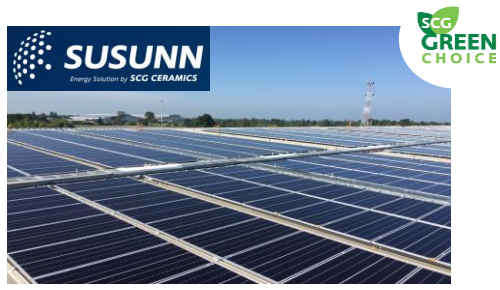
SUSUNN electricity produced by PV system
