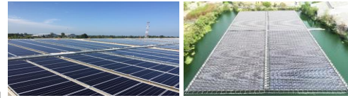
Solar floating Solar rooftop
