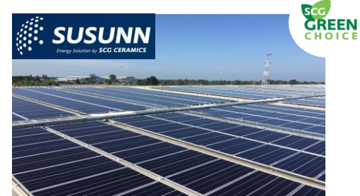
SUSUNN electricity produced by PV system
