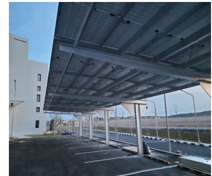
Southern Industrial Estate Songkhla Provincial (SEZ) 42 Kwp
