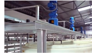
Water Treatment & Water reuse
