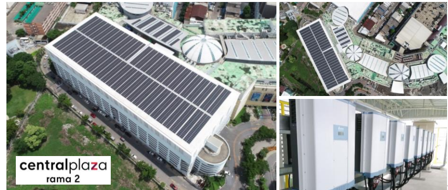
CPN at Central Plaza Rama II 998.8 kWp
