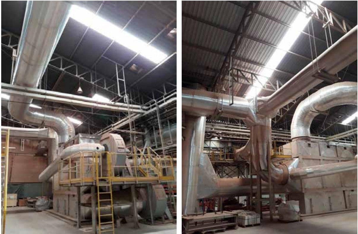
Waste Heat Recovery from Kiln's Chimney (Air to Air Heat Exchanger )
